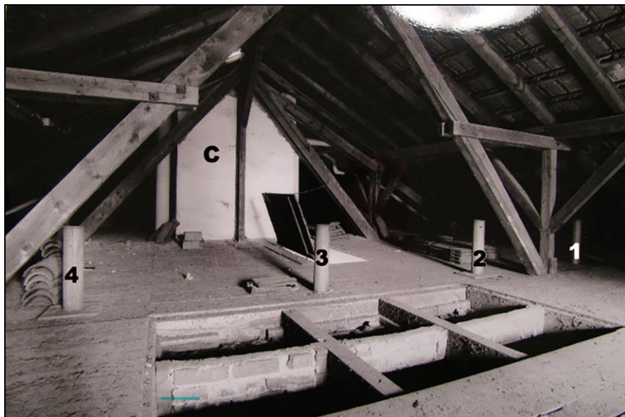
Document 34: Photo by R. Müller showing the attic of the Dachau crematorium above the boiler room (1995). Source: Archives of the Dachau Museum, Folder Krematorium Baracke X.
