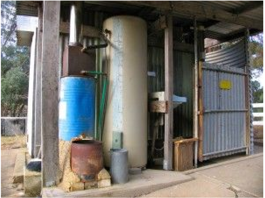
Rocket stove connected to a water tank.
