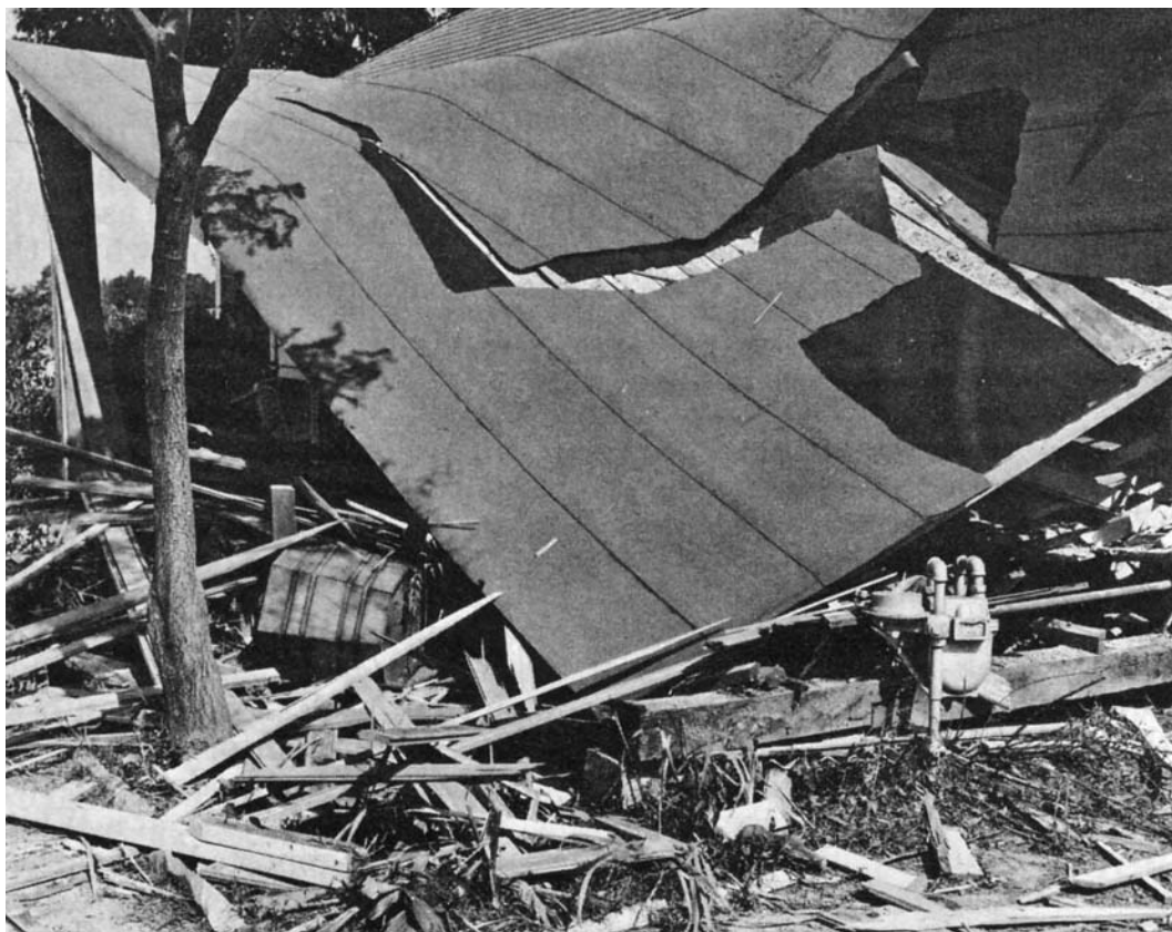
A Klan bomb wrecked the home of Aylene Quinn in McComb on 20 September 1964 (HCUA).
