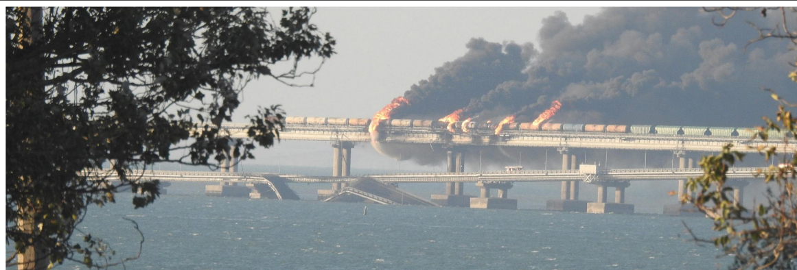
Damage to the Crimean automobile bridge, train of fuel cisterns can be seen burning on the railway bridge.
