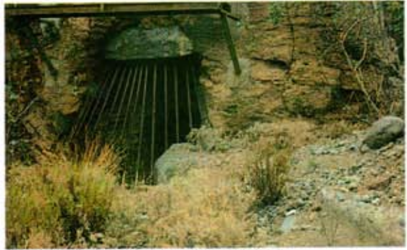
61. LAS PALMAS, CANARY ISLANDS. An arroyo is part-blocked by concrete/stone barrier on right, and bled off via a coarse trash screen to tunnels ( galeria ) and cave storages linked to irrigation systems at lower levels.
