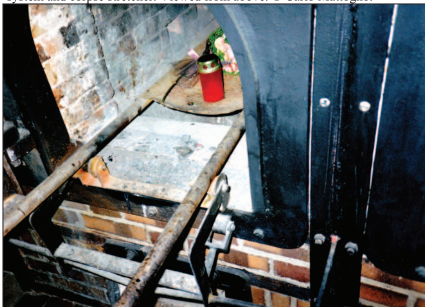
Document 45: Crematorium of Mauthausen. Topf coke-fired double-muffle, oven Auschwitz type. Loading system of oven: fixation shaft, mobile roller device supporting the bars of the corpse stretcher. © Carlo Mattogno.
