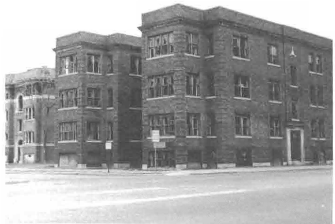
Wrecked, vandalized and abandoned apartments
